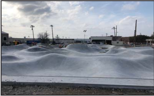
The new skate park downtown at Porter and Third streets is nearing completion.
